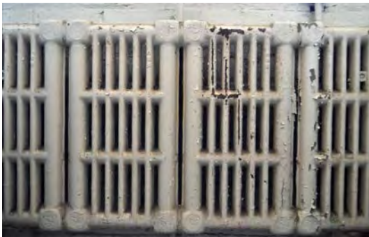
Figure 8. A cast iron radiator.
