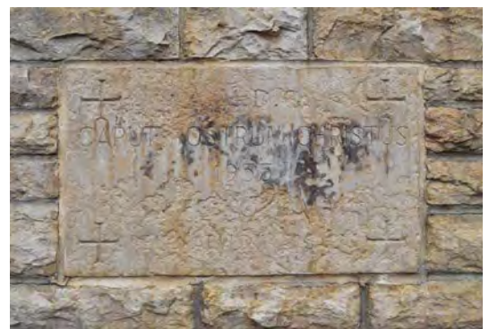
Figure 50. The cornerstone, showing signs of weathering.
