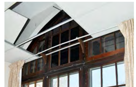
Figure 15. A gothic arch window. The arched transom has been hidden from view on the interior by a dropped ceiling. Stucco on obscures the window on the exterior.
