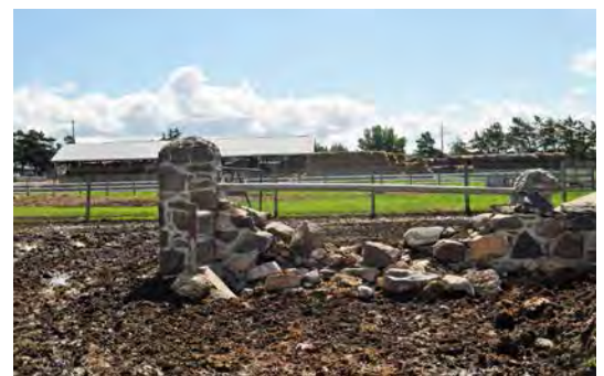
Figure 5. A portion of the stone fence which has fallen down.
