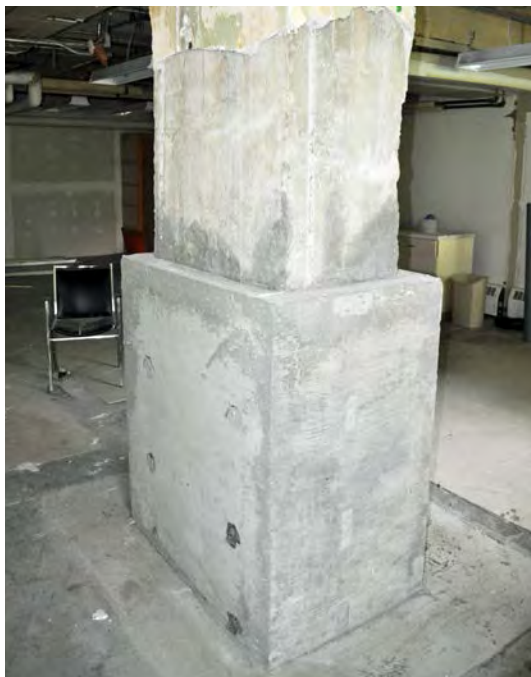
Figure 23. Concrete columns in the basement have been underpinned to address structural degradation.
