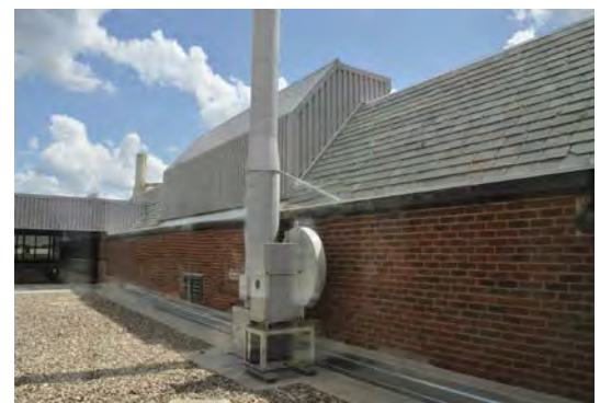
Figure 6. Roof materials: slate tiles for sloped portions and membrane roofing for flat portions.
