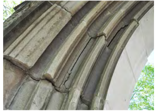
Figure 3. Indiana limestone showing signs of deterioration.
