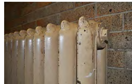
Figure 7. Cast iron radiator.
