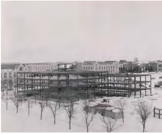
Figure 19. The steel structure of the Murray Building, winter 1954-1955. Photo A-597, retrieved from http://sain.scaa.sk.ca/items/index.php/university-of-saskatchewan-archives;isdiah
