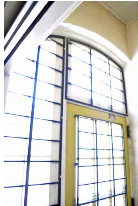
Figure 9. Steel bars have been retrofitted over the interior side of the windows.
