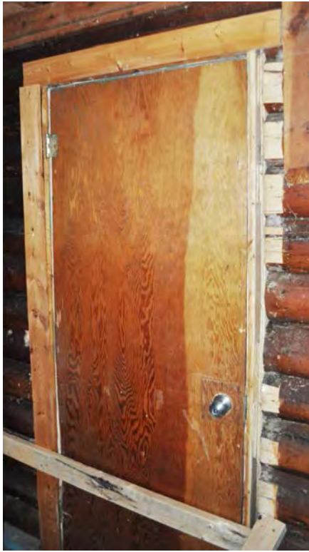
Figure 8. Damage due to vandalism.
