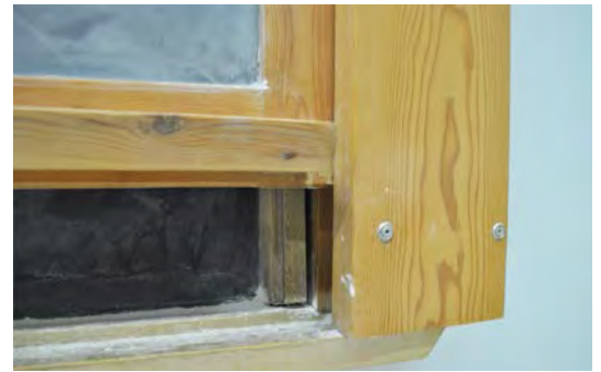
Figure 12. Slate chalkboard beneath a newer chalkboard that has been added over top.
