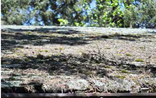
Figure 7. State of roofing material.
