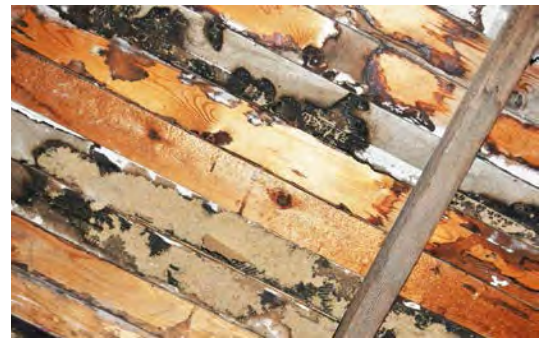
Figure 5. Fir roof decking showing signs of water ingress.
