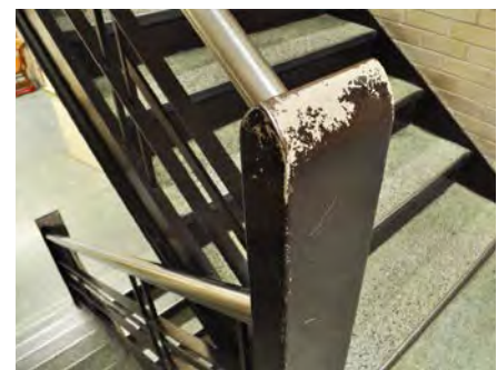
Figure 12. Staircase materials: steel stringers, risers and balustrade with terrazzo treads and landing.
