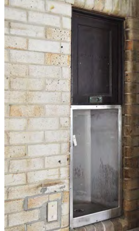
Figure 8. Remaining wood panelling over replaced sink.
