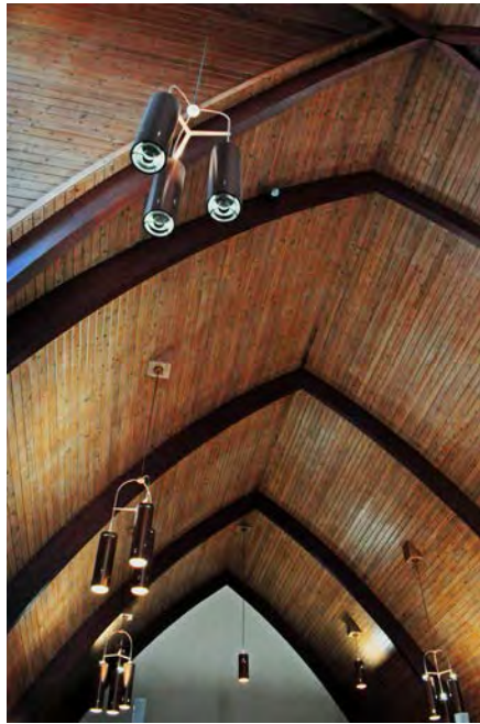
Figure 13. Light fixtures in the chapel's nave.
