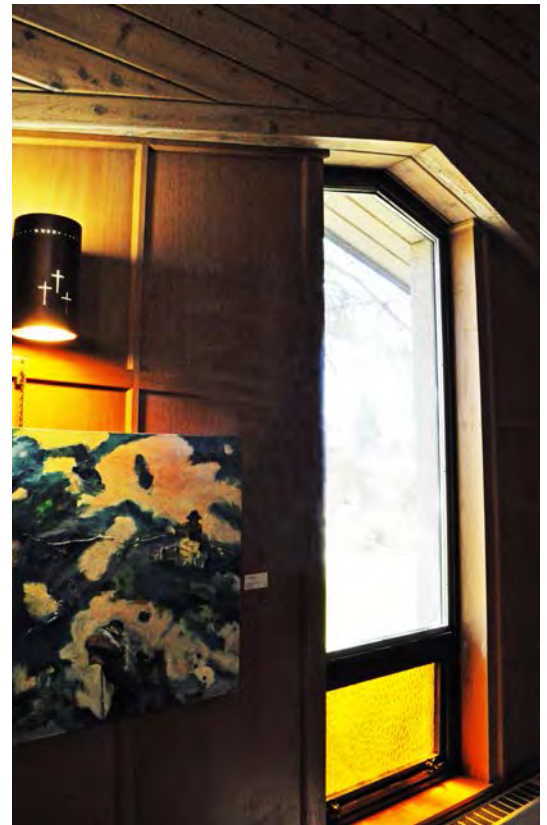
Figure 9. This window is modern in style but its peak pays tribute to the gothic style.
