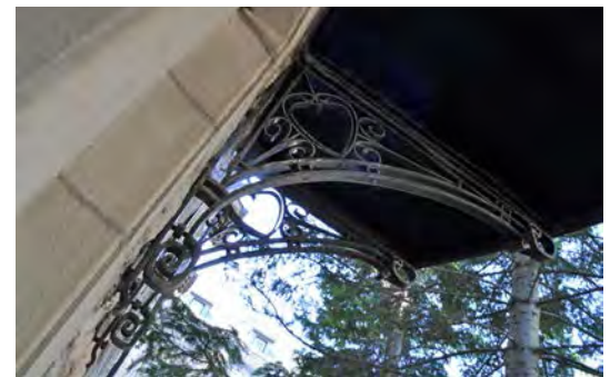
Figure 4. Steel brackets supporting a balcony on the west side of Qu'Appelle Hall.
