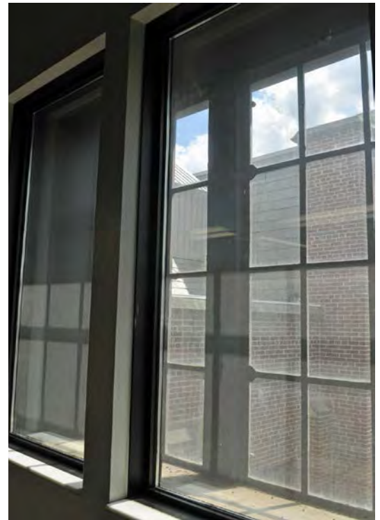
Figure 4. New aluminum framed double glazed windows have been fitted over the interior of the original windows.
