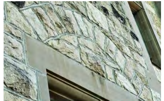
Figure 36. A stone relieving arch helps to support the wall over a window.
