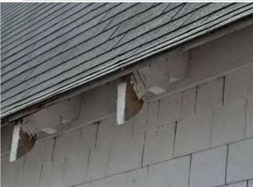
Figure 2. Top to bottom: Asphalt roof shingles have replaced the original cedar shingles, carved exposed wooden truss ends. The cedar shakes on the upper portion of the main barn have been painted white.
