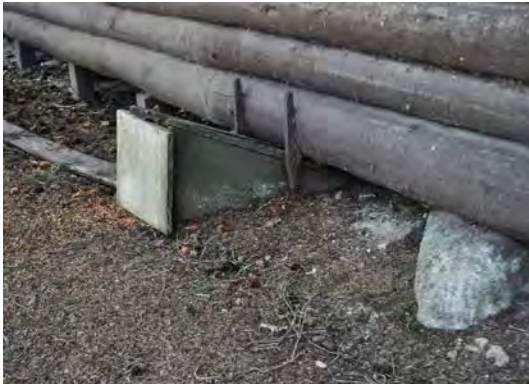
Figure 15. L to R: coal chute and a rock supporting the cabin's base.
