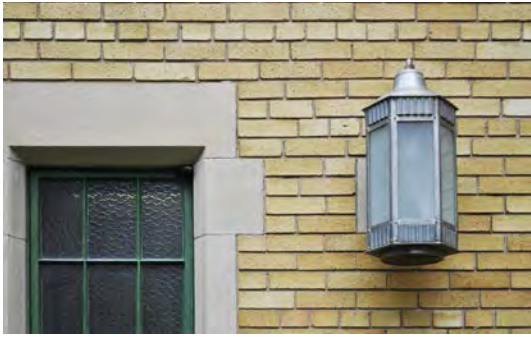
Figure 7. Exterior window materials: steel sash window, limestone surround and yellow brick wall.
