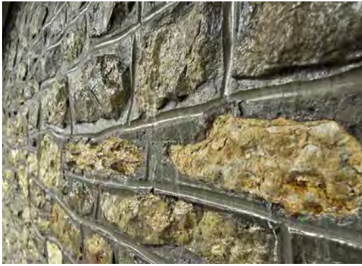
Figure 3. A greystone wall which now forms part of a basement meeting room.
