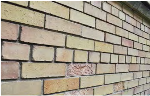
Figure 1. Yellow brick showing some spalling.
