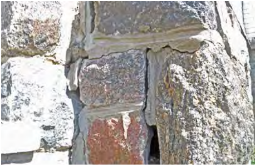
Figure 21. Deterioration of the walls of the Stone Barn.
