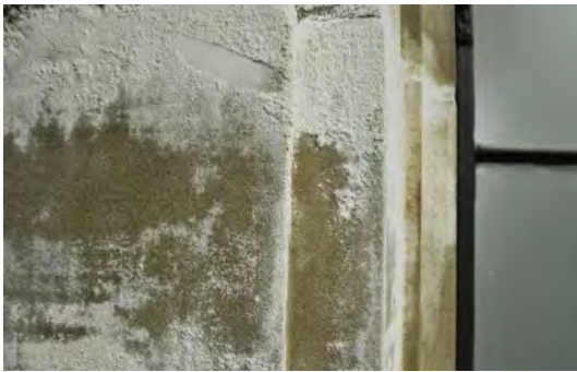
Figure 4. Stone with efflorescence.
