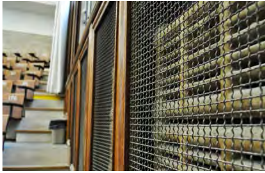
Figure 12. Painted cast iron radiators in original oak cabinet with brass screen.
