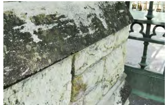
Figure 4. Limestone showing surface staining and corrosion.
