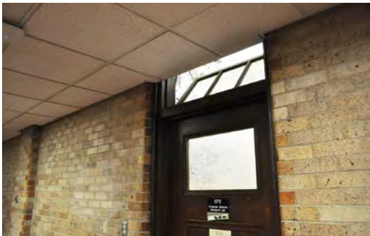
Figure 21. Transoms in the basement have been compromised by a dropped ceiling.
