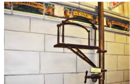
Figure 28. Non - functioning fire hose carrier.
