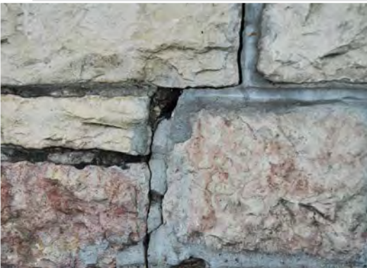
Figure 1. Greystone showing signs of deterioration in the mortar joints. The right half of the photograph shows an attempted repair using inappropriate material.
