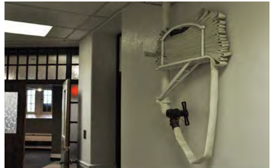
Figure 55. Fire hose apparatus.
