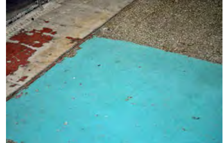
Figure 8. Marble and terrazzo located around the former pool. Both show evidence of having been painted.
