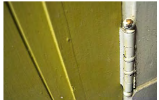
Figure 5. A brass hinge on a wooden door, both of which have been painted.
