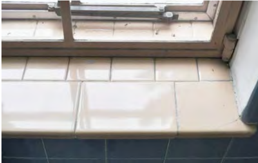
Figure 9. Buff and blue ceramic tile under a steel casement window in the 1959 wing.
