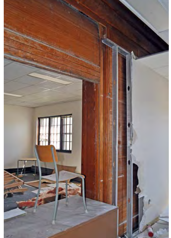
Figure 5. This coiling partition made of Douglas Fir was covered by gypsum board in 1992.
