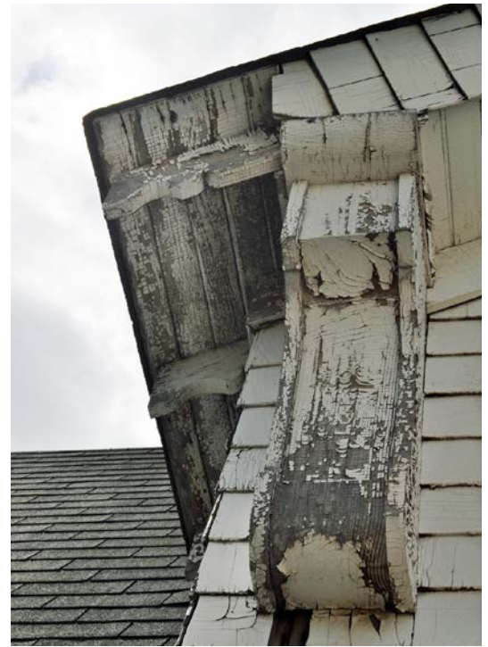
Figure 12. Carved wooden brackets flank the ramp doorway and carved wooden rafter extensions are visible under the eaves.
