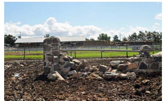
Figure 5. A portion of the stone fence which has fallen down.
