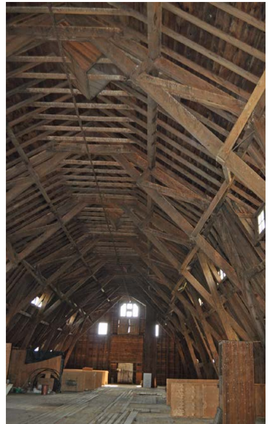
Figure 8. The loft features unfinished Douglas fir. The lower right corner shows a ventilation shaft that has been disconnected from a cupola. The opening for the cupola can be seen at the top left of the photograph.
